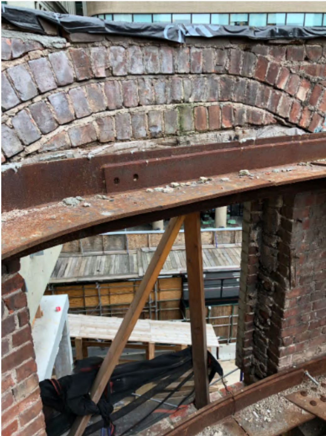
A close-up shot of the arched bricks for the upper windows and the steel frame that holds up the exterior. Photo by Michael Young
