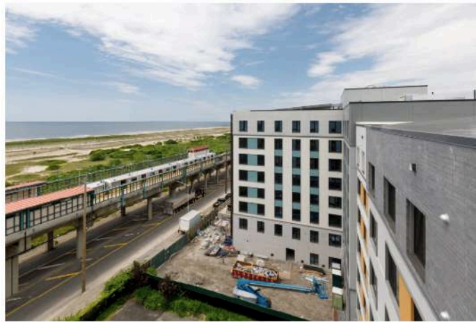
Climate change is a real concern on the Queens shoreline that Hurricane Sandy ravaged in 2012. Beach Green Dunes will have resiliency measures, like an elevated patio that doubles as an emergency boat dock, and green energy features.
