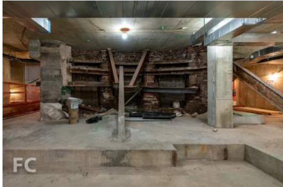
Foundations of the Robert & Anne Dickey House integrated into the new structure's cellar level.
