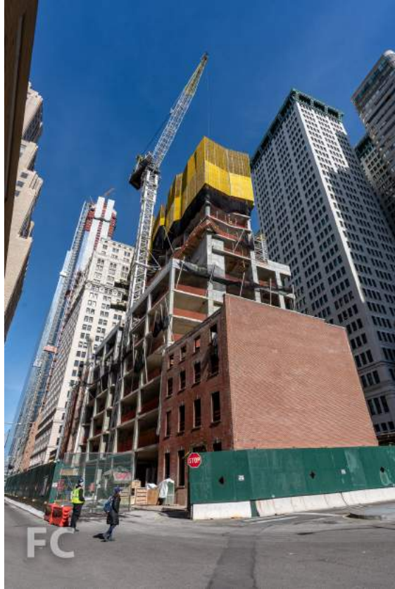
Looking up at the southwest corner of the tower (left) and the Dickey House (right).
